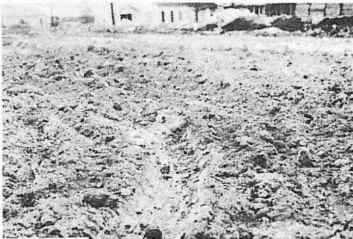
By 5:00 p.m. the wet clay has dried out sufficiently for compaction to proceed. The compacted lime-treated subgrade will provide excellent support for the concrete floor slab.
