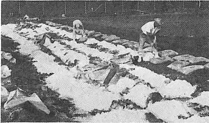
Workers slit open bags and dump hydrated lime in piles at Texas Highway Department warehouse site, Bryan. Note how lime blots up moisture from saturated clay soil.
