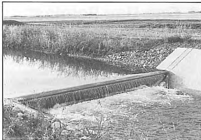
Concrete weir checks water at low flow in the Chin 2 Lateral.
